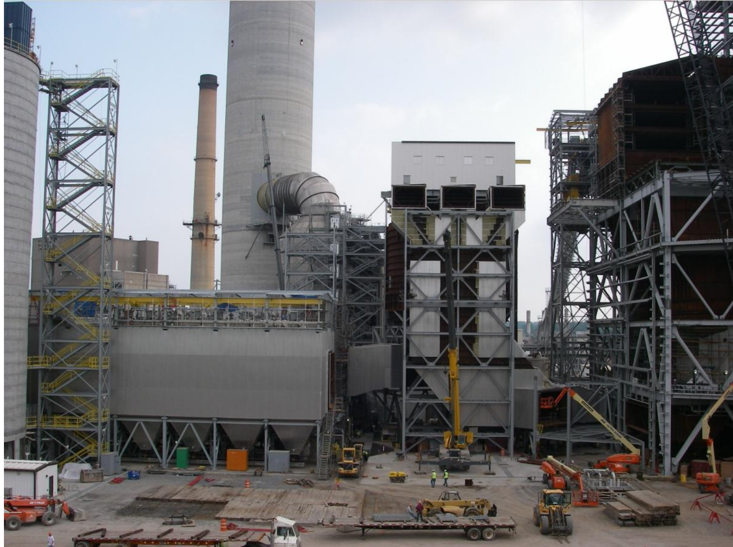
Cliffside 6 Integrated AQCS - July 2011
